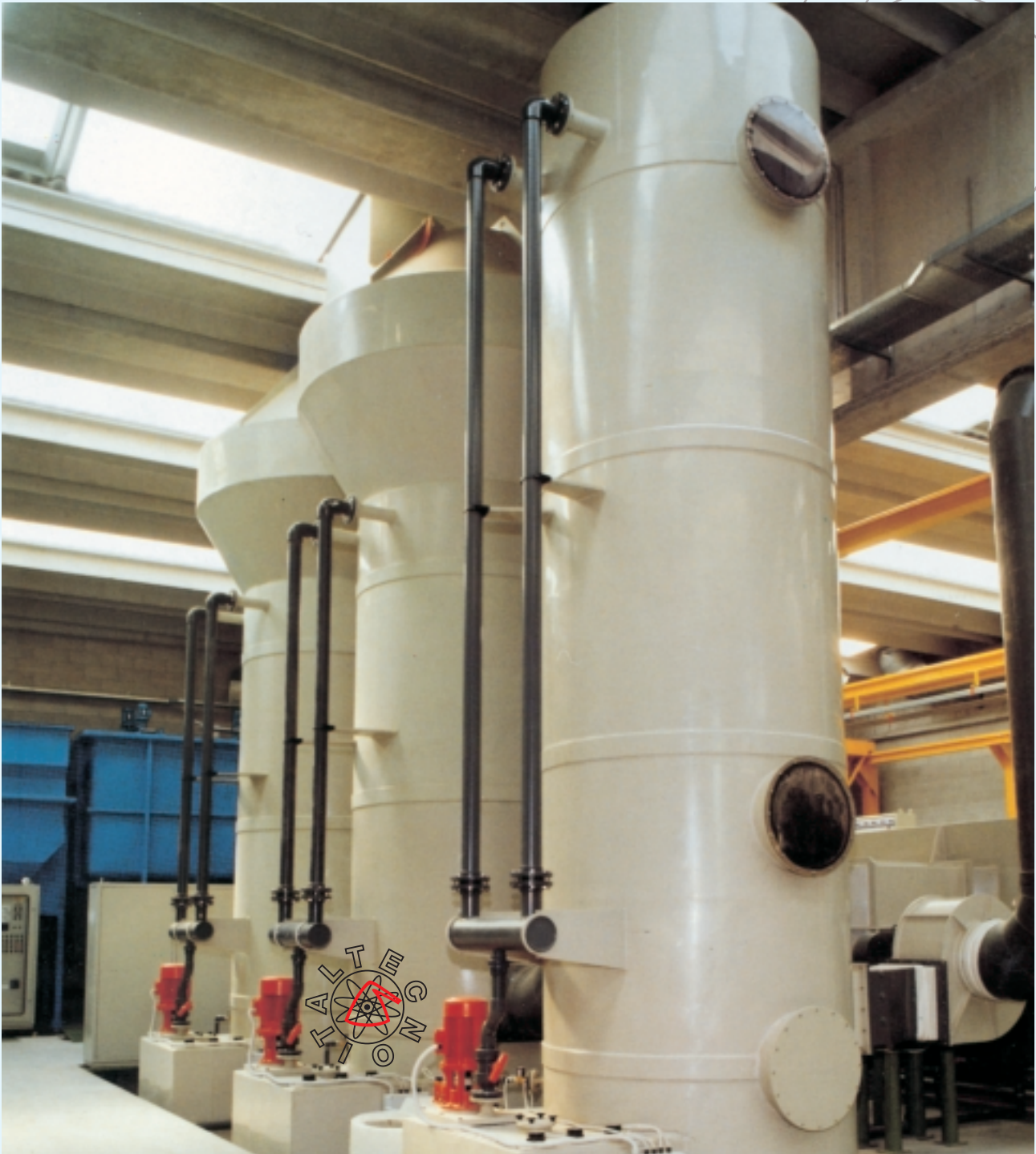
Example of neutralization towers for expulsion of fumes treated to guarantee conformity with local environmental regulations governing emissions.
